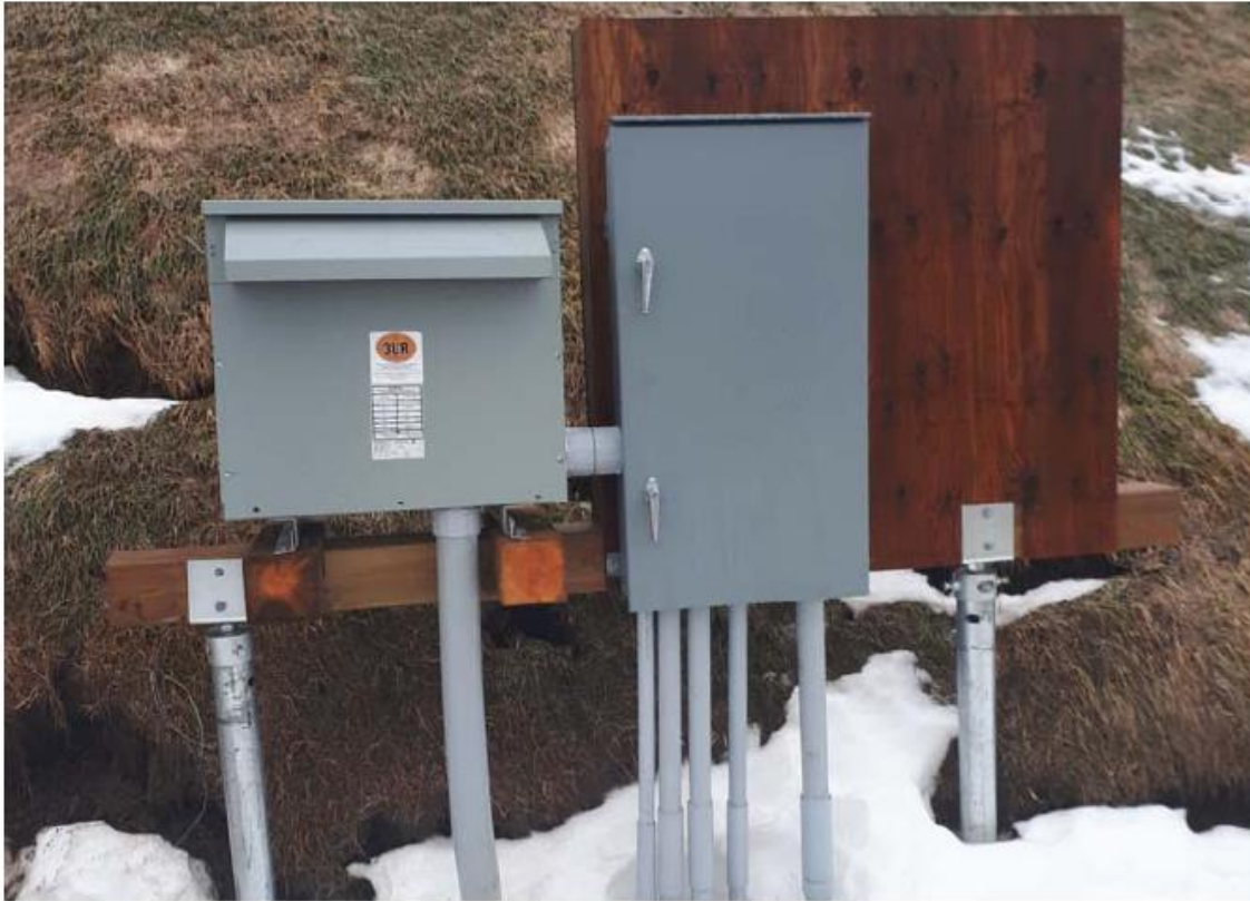
Photo 6 - Electrical Box at North Berm
